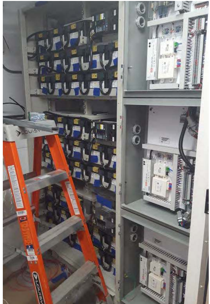
Fig. 6: MEG Factory Build Battery Racks
