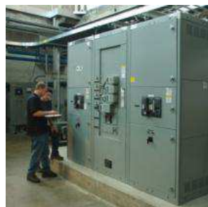
Switchgear up to 1300 KW
