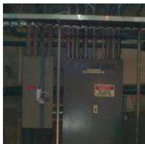
2.5MVA Grid Interconnect
