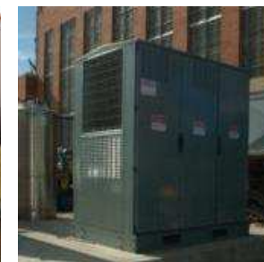
Load Bank 400 KW 0.8 PF
