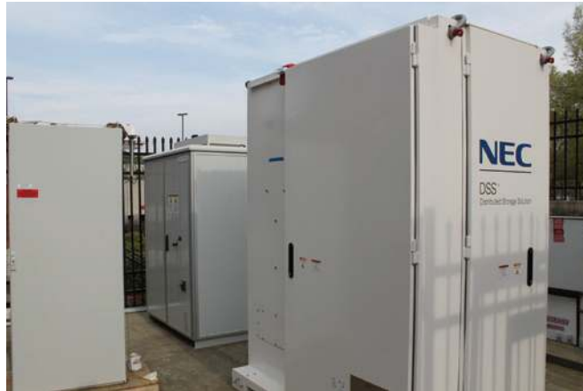
Figure 1: BESS and Controller.
